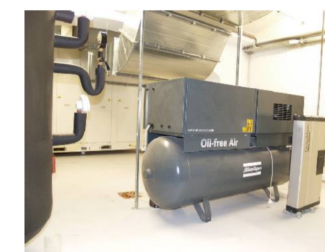
Air supply Cooling system
